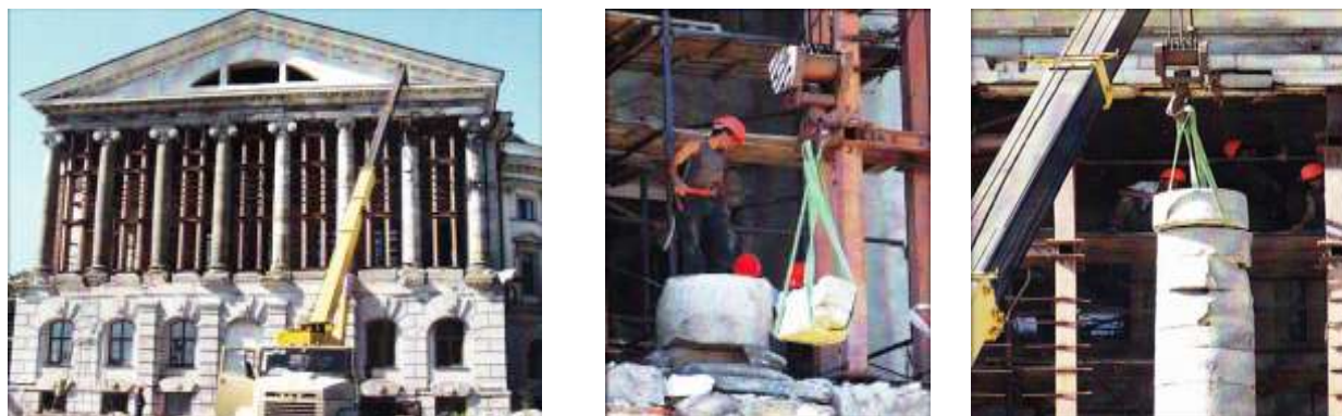
Fig. 7. Installation of columns of the southwestern façade of the palace of K. Razumovsky (2008).
